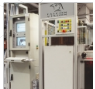
In-line measurement system
